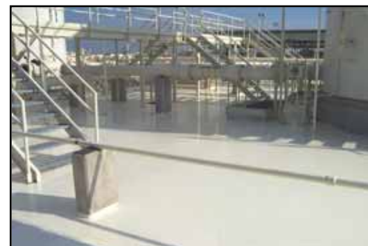
Containment site protected with EPI's system of Joint Sealant, Quick Set Epoxy and RAP 45 Aliphatic Polyurea decreases the environmental risks posed by stored hazardous materials.
