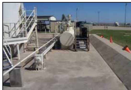
Containment site before placement of EPI coating system. Photos courtesy of Weston Solutions, Inc.
