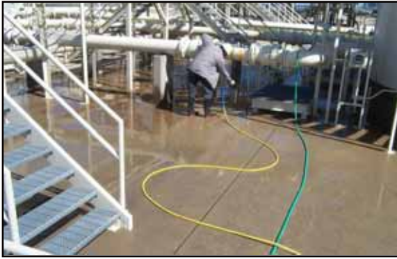
Surface preparation is critical to remove all contaminants and to repair all leaks and cracks.
