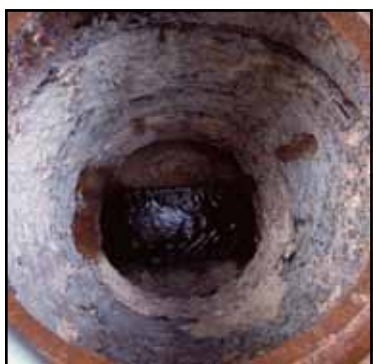
A typical scene showing corrosion and structural deterioration before an application of EPI's silicone-modified polymers
